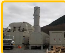
Houses Backup Diesel Generators
