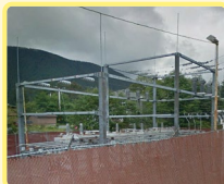
Marine Street Substation
